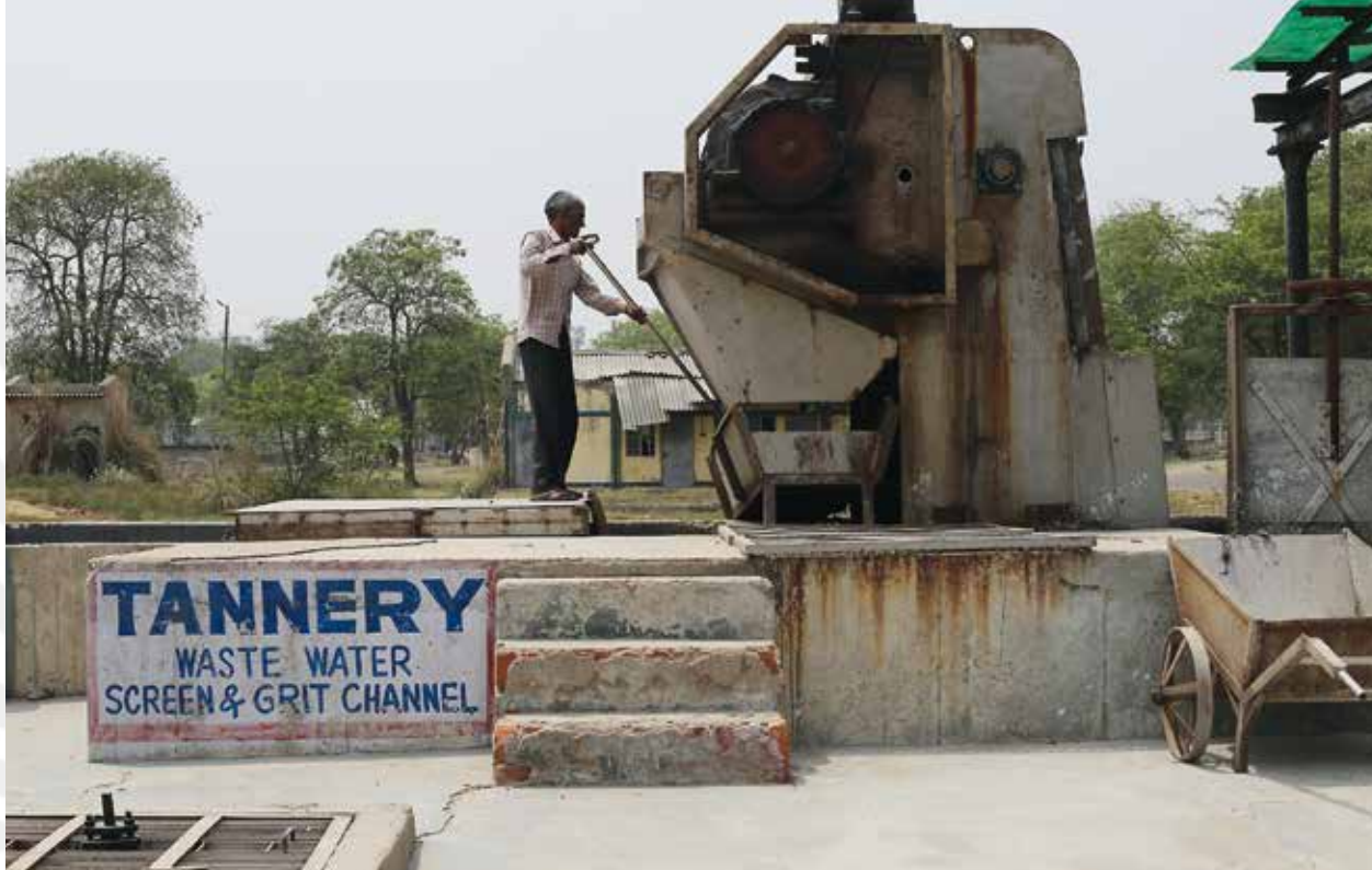
Common Effluent Treatment Plant (CETP) in Kanpur treating tannery wastewater
